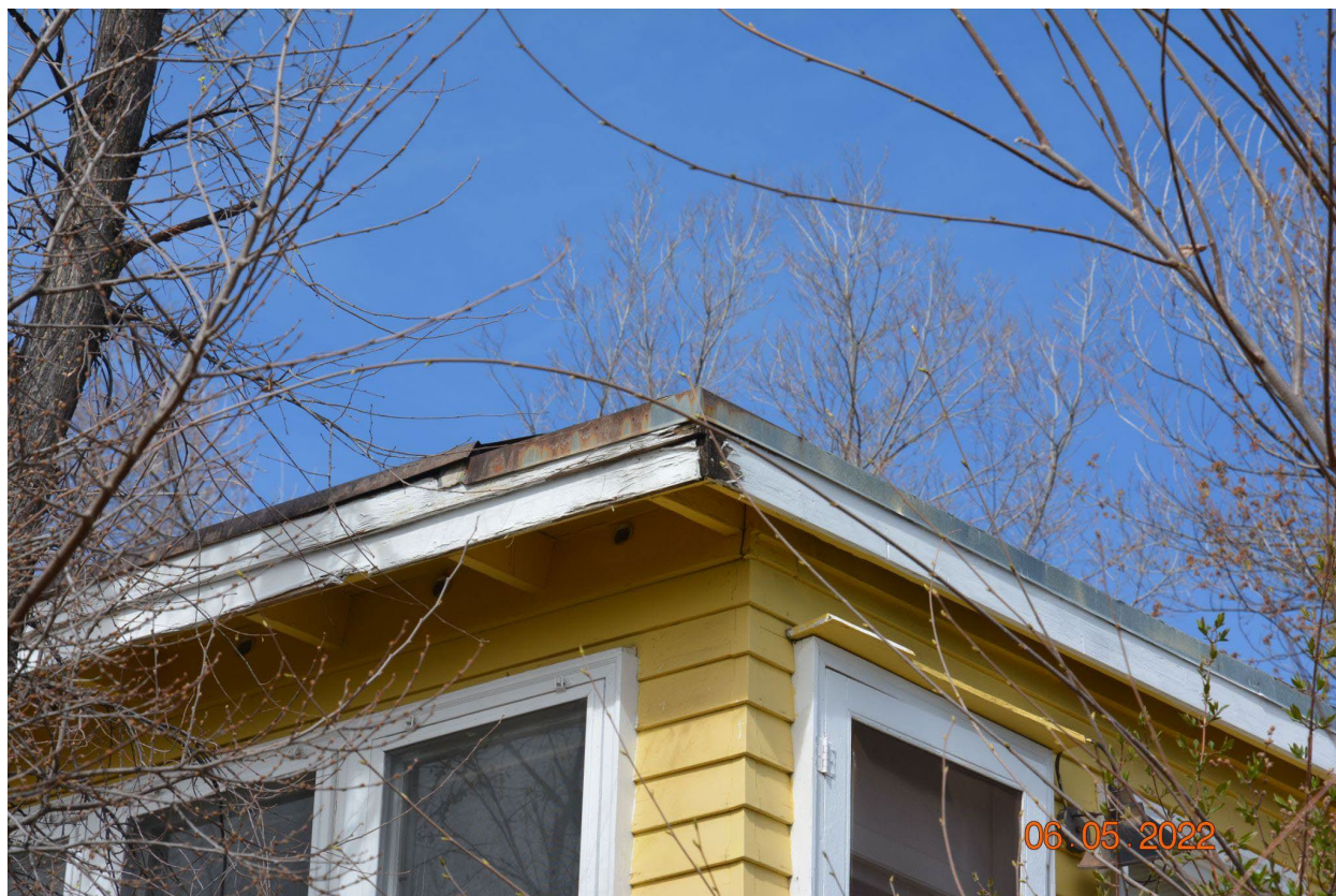
Figure 7. Deteriorated fascia board that provides an entry for wind-blown embers can result in an ignition on the interior of the structure.
