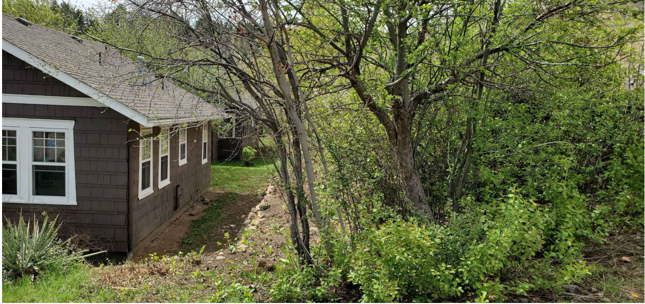
Figure 3. Western boundary where fuels mitigation is yet to be conducted. Note the horizontal and vertical continuity of the vegetation which would allow for a fire to easily spread.
