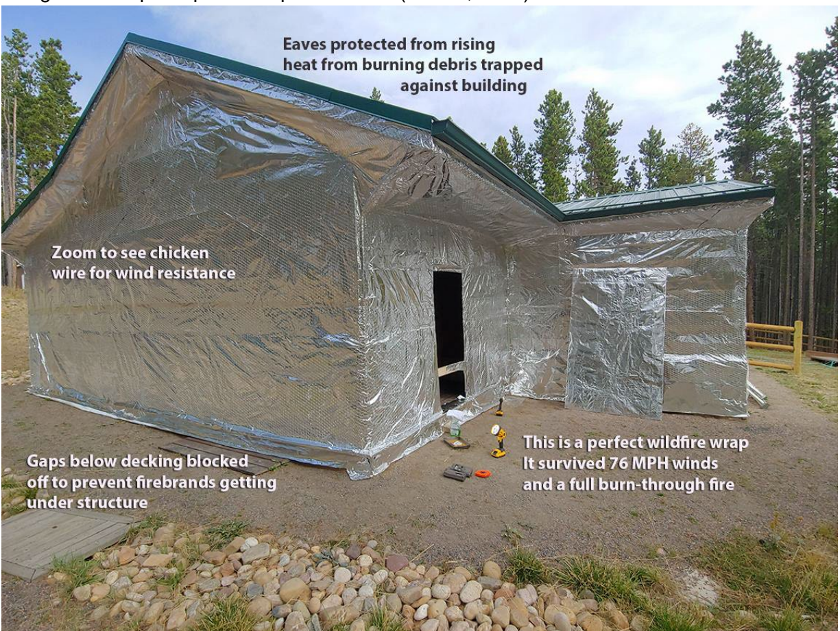
Figure 10: Firezat installation with chicken wire and staples. Building has an existing metal roof eliminating the need to wrap the roof. Image credit: firezat.com, accessed March 21, 2023
