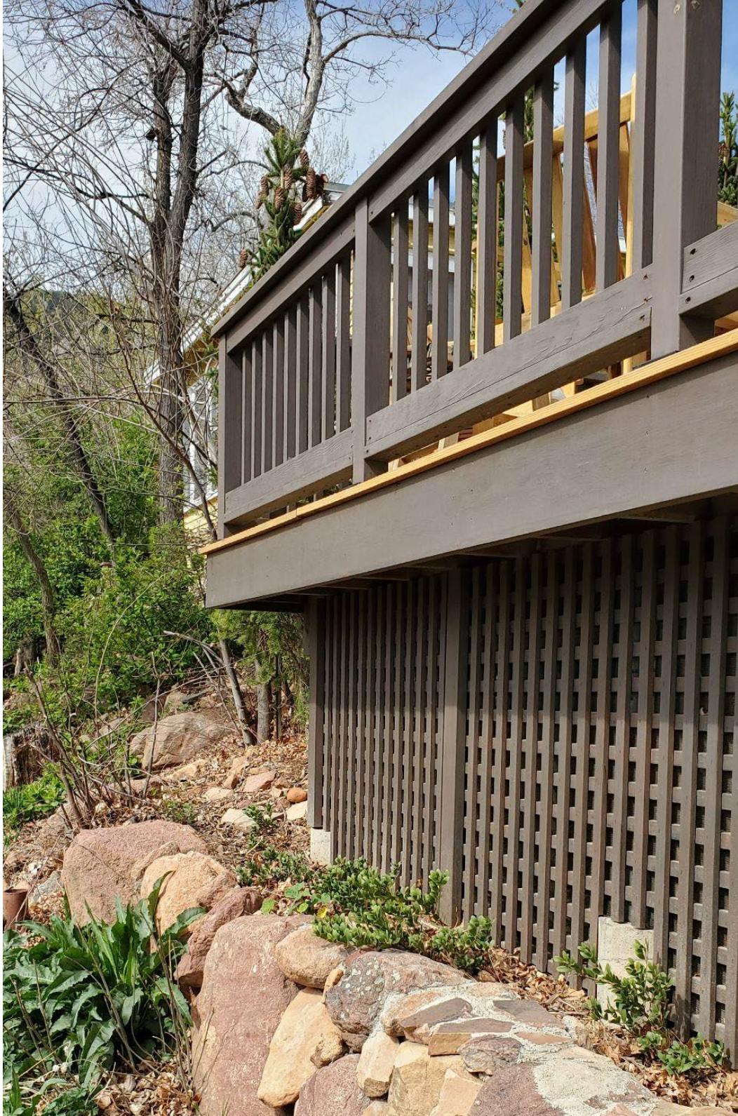
Figure 13. Mary H. Galey Cottage deck enclosure. The enclosure uses fire-retardant-treated wood and metal mesh to reduce combustibility and the likelihood of large embers causing ignition under the deck.
