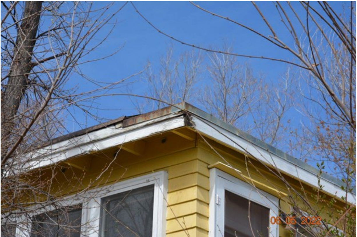
Figure 8: Deteriorated fascia board that provides an entry for wind-blown embers can result in an ignition on the interior of the structure.
