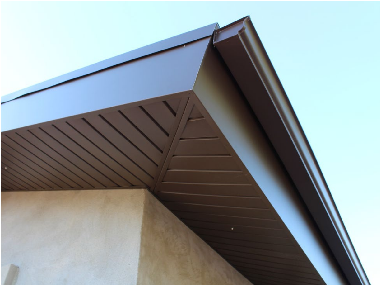
Figure 20: A Plus Gutter Systems of Los Angeles and Orange County, Photo of soffit and fascia retrofitting with sheet metal, Accessed May 17, 2023
