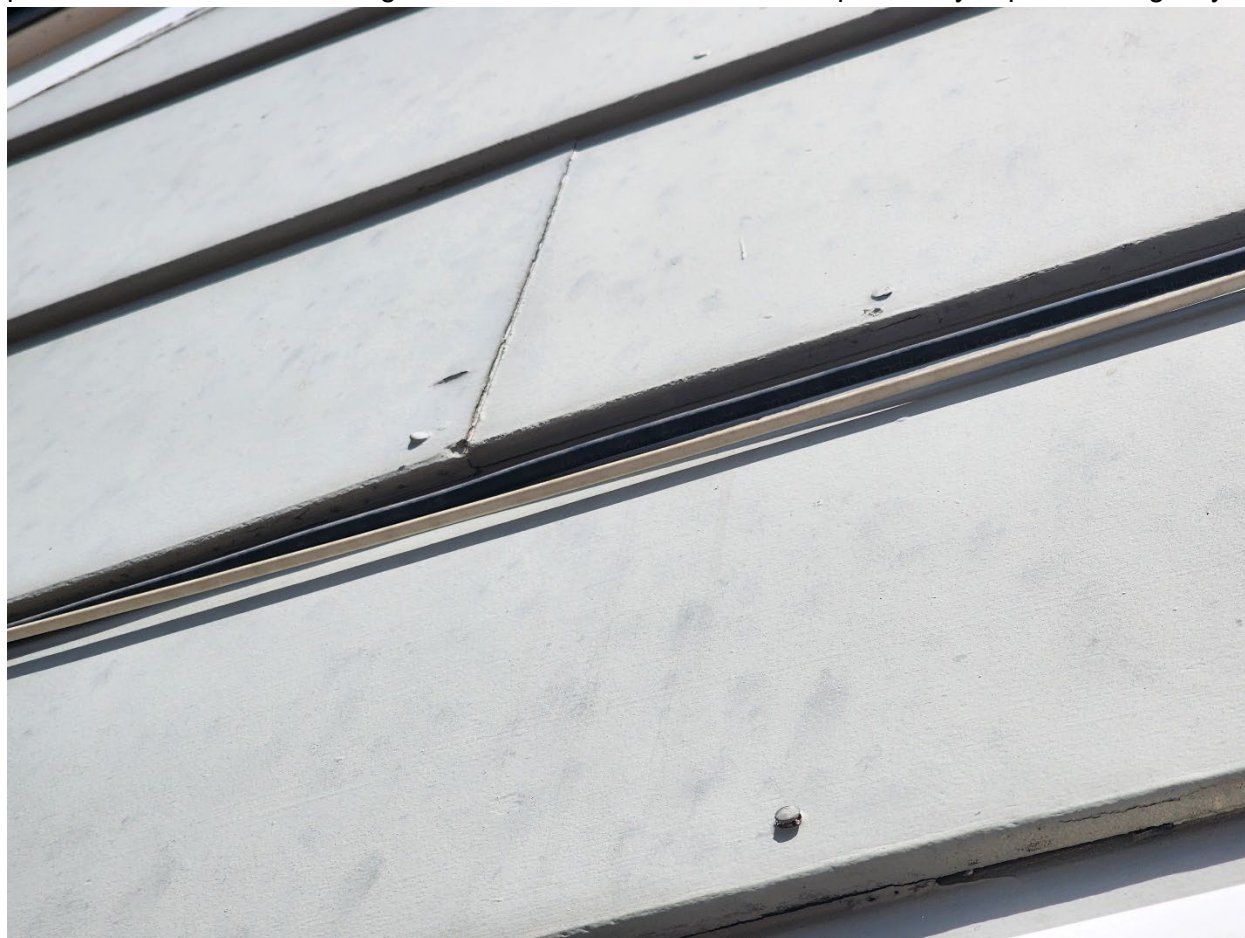
Figure 34: West Wall of 1957 Ranch in Colorado, Nails Visibly Working Their Way Out of Fiber Cement Siding (Lord, 2023)
