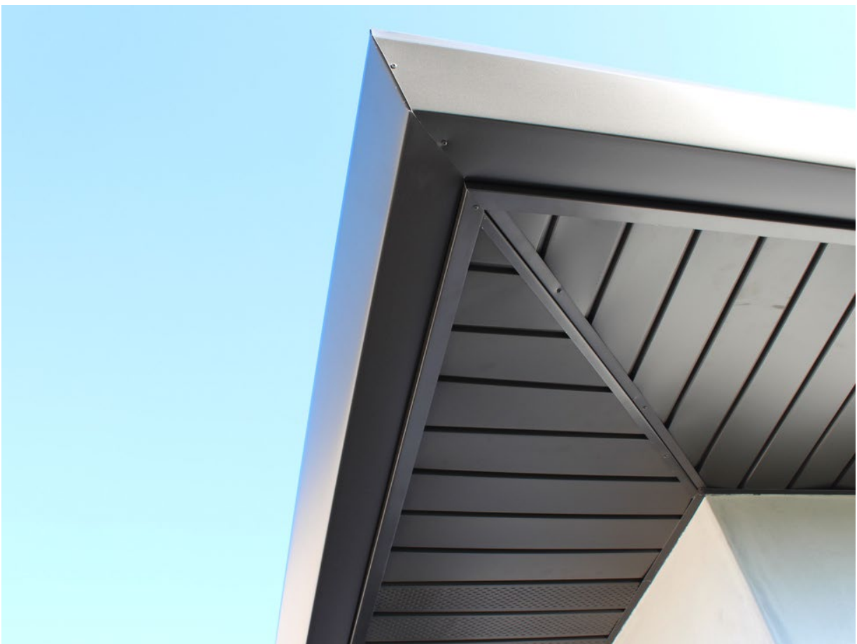
Figure 19: A Plus Gutter Systems of Los Angeles and Orange County, Photo of soffit and fascia retrofitting with sheet metal, Accessed May 17, 2023
